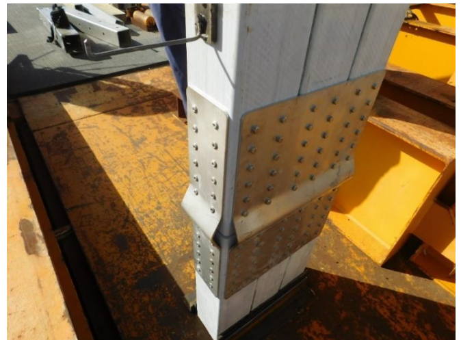
Figure 8. Failure mode of the tested sample
